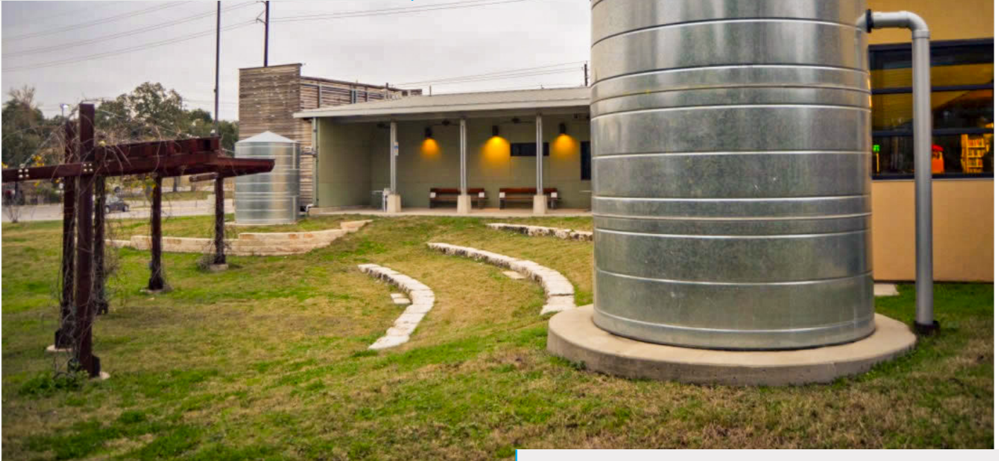
Two 2,500-gallon cisterns sitting at the back corners of the library. Photo Credit: Texas Water Development Board
