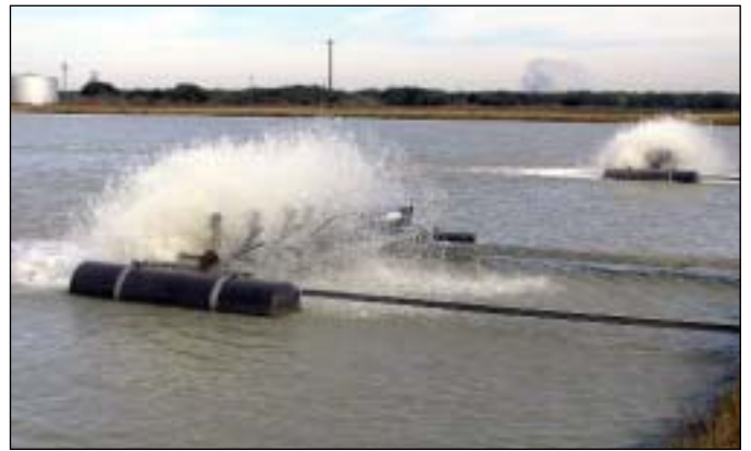
Figure 16. Electric paddlewheel aerators.
