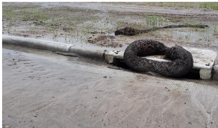
Figure C- 2. Example of a failing stormwater BMP; Photo taken just north of the watershed
